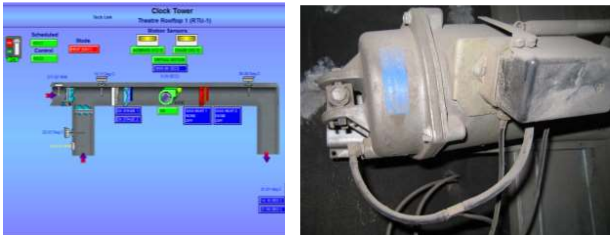
Figure 8: Theatre Rooftop Unit – DDC Graphic & compressed air damper actuator
