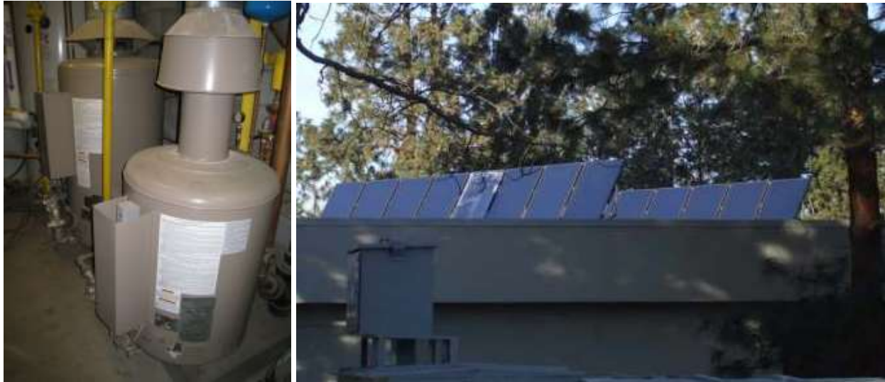
Figure 7: Culinary Arts Domestic Hot Water Boiler and Solar Hot Water Panels
