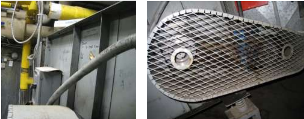
Figure 16: AHU-F6 and AHU-F13
